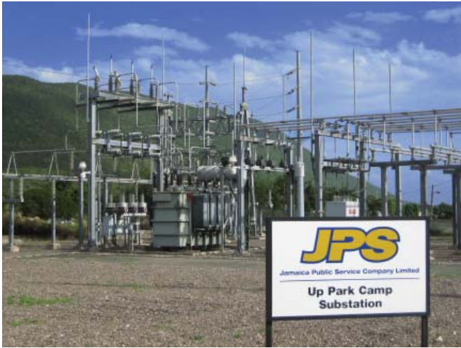
Up Park Camp substation in Kingston
